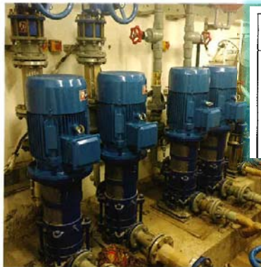
The new motor of potable and flushing water up-feed pump has been installed
